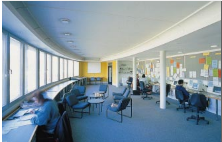
An IT resource room is located directly above the main entrance, and follows the gentle curve of the elevation. Note the row of annular soffit diffusers connecting directly to the exposed Termodeck slabs.
